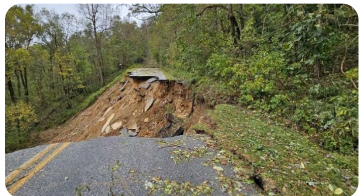
Figure 3: Landslide Damage to Gooch Gap at Milepost 336
