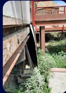
Support damage to portable school building.
