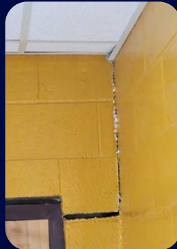
Cracks in Building 621.
