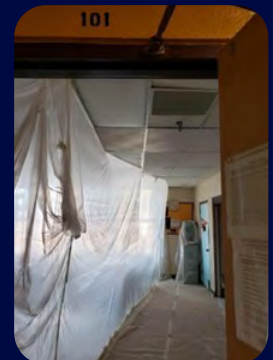
Damage and repairs from a sewer break.
