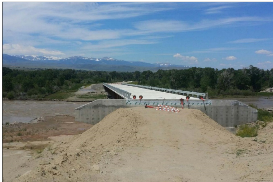
Figure 1. The Lenore Bridge project has not been completed, as the approaches still have not been constructed. Source: OIG.
